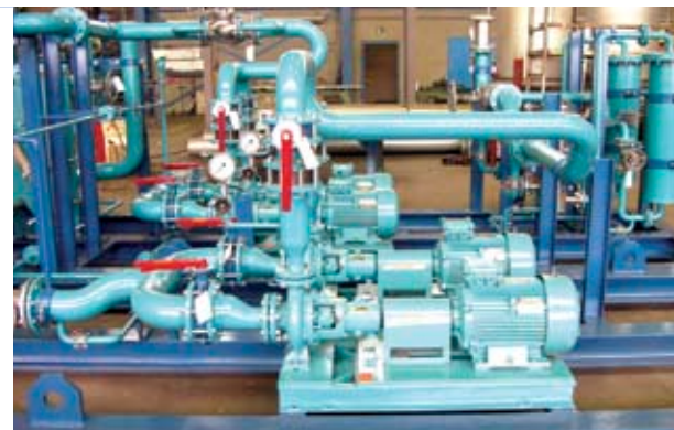
Pump and filter station for MEA-solution
